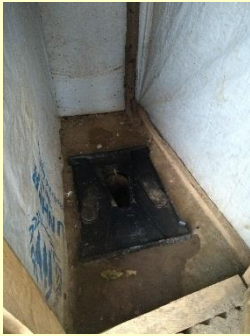
Figure 26 - Current latrines with plastic slabs. Note fecal material on slab.
