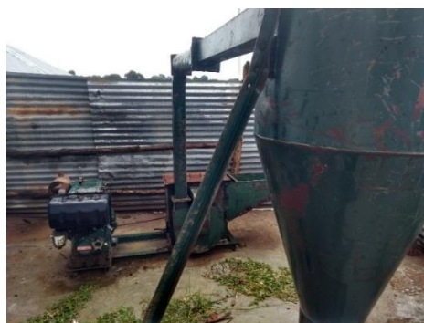
Figure 16 - Grain mill livelihoods project in Ariwa decommissioned from lack of maintenance.
