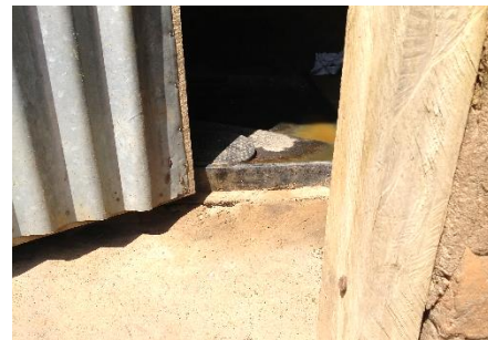
Figure 43 – Latrine slab interference prevented basins from passing through the doorway.
